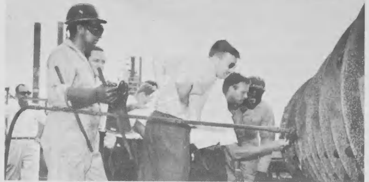
Demonstration (top picture) is given on how tube bundles are cleaned by high pressure water jetting. Closer inspection (lower picture) shows result of cleaning using just water.
